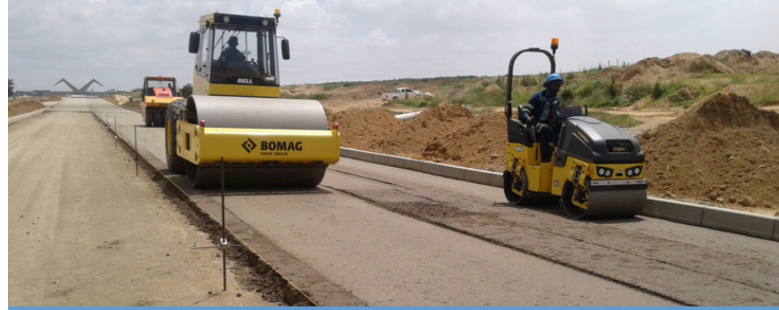
William Nichol Drive: Compacting micaceous G5/G6 with nano-technology product added for the Gauteng Province Department of Roads and Transport (GPDR).
